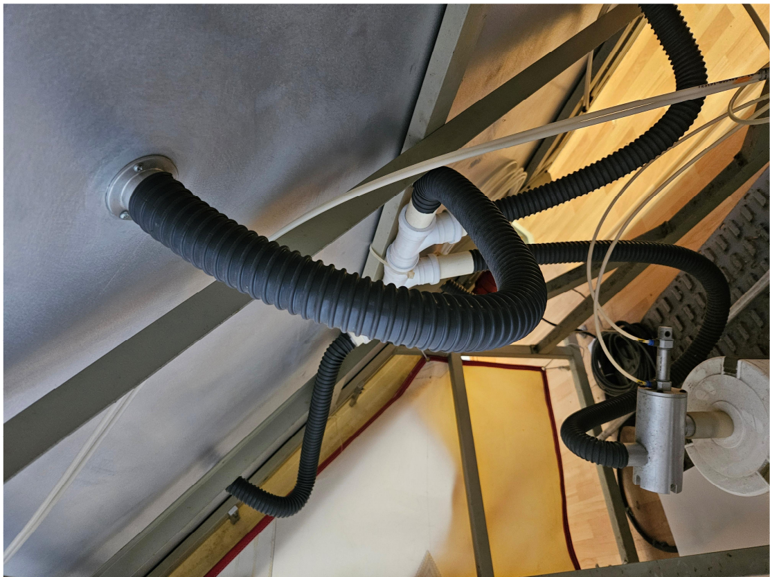
Figure 9: Sailmaking Plotter, closeup of plumbing.
