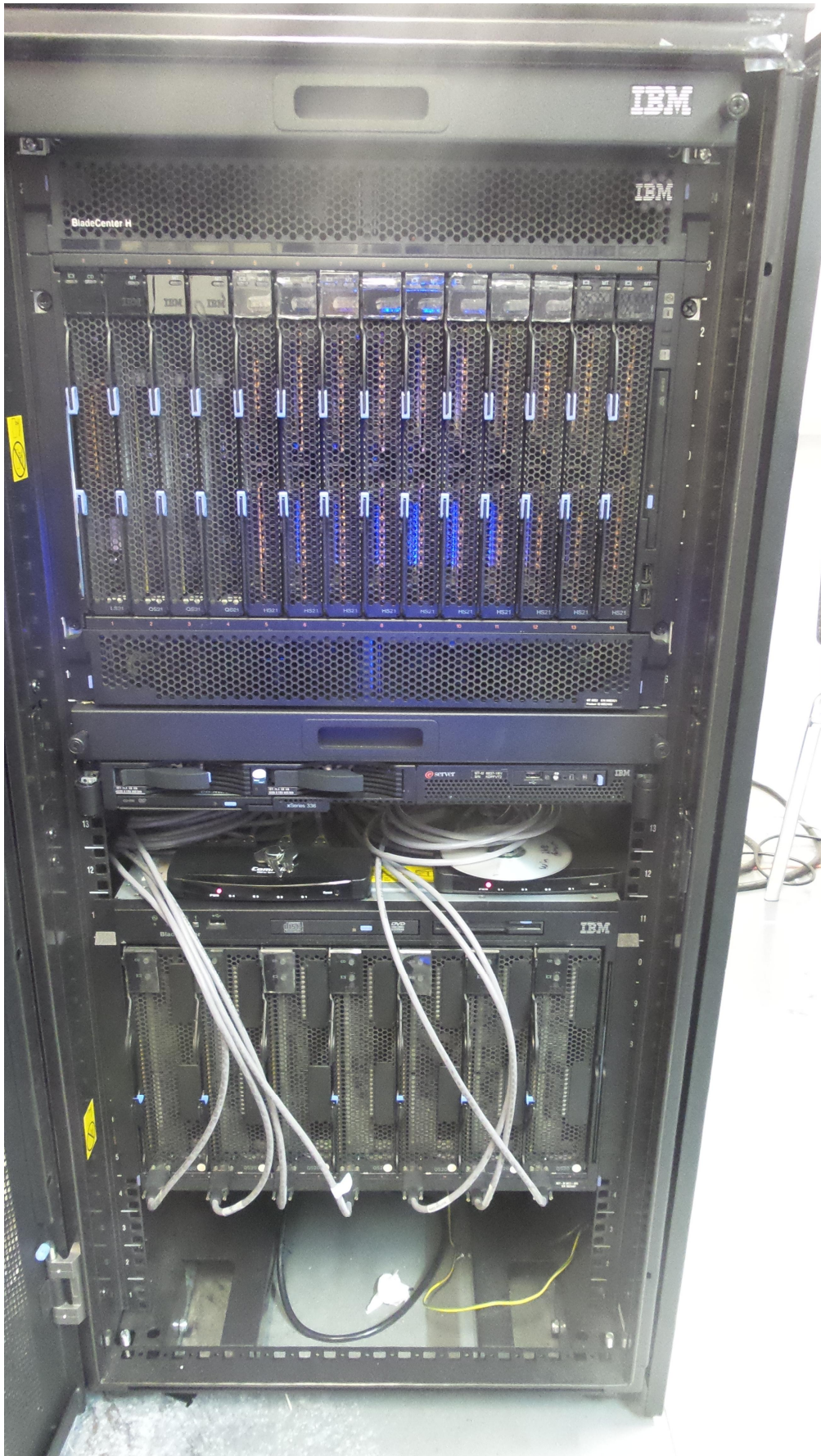
Figure 2: IBM BladeCenter QS20 front view
