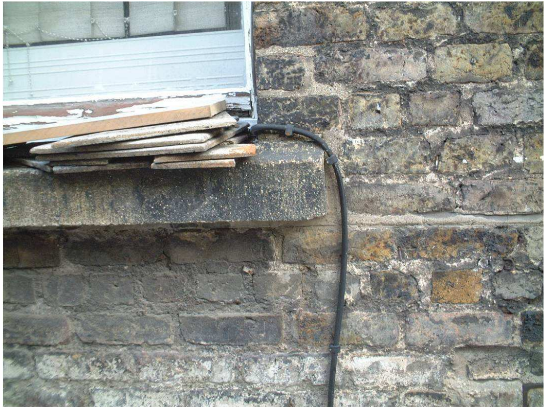
Figure 76: 3Mbps Ethernet cabling at Dept. Computer Science, TCD Photo courtesy Mike Nowlan
