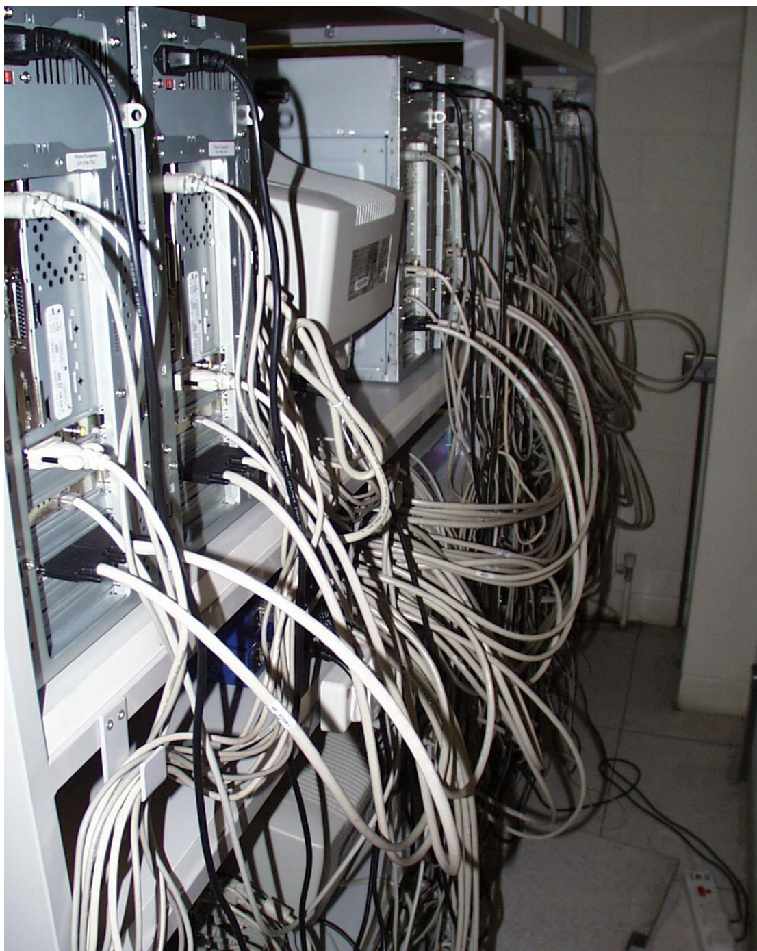
Figure 4: CAGcluster0 rear view showing SCI and Ethernet wiring
