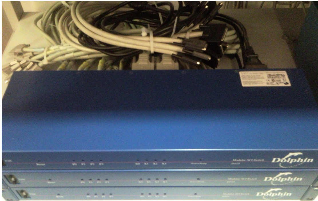
Figure 5: CAGcluster0 SCI switches after removal, again showing SCI wiring
