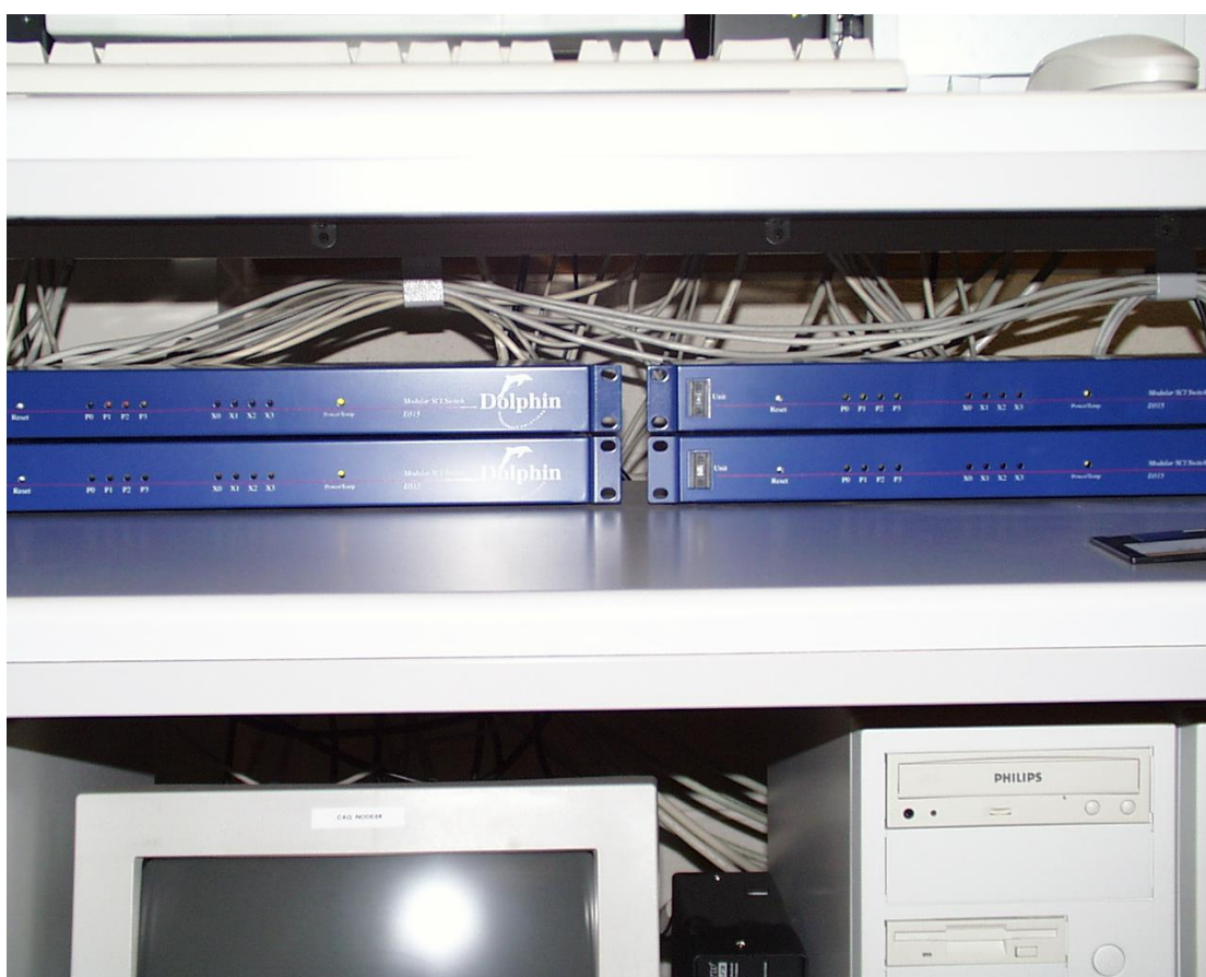
Figure 3: CAGcluster0 front closeup showing SCI switches
