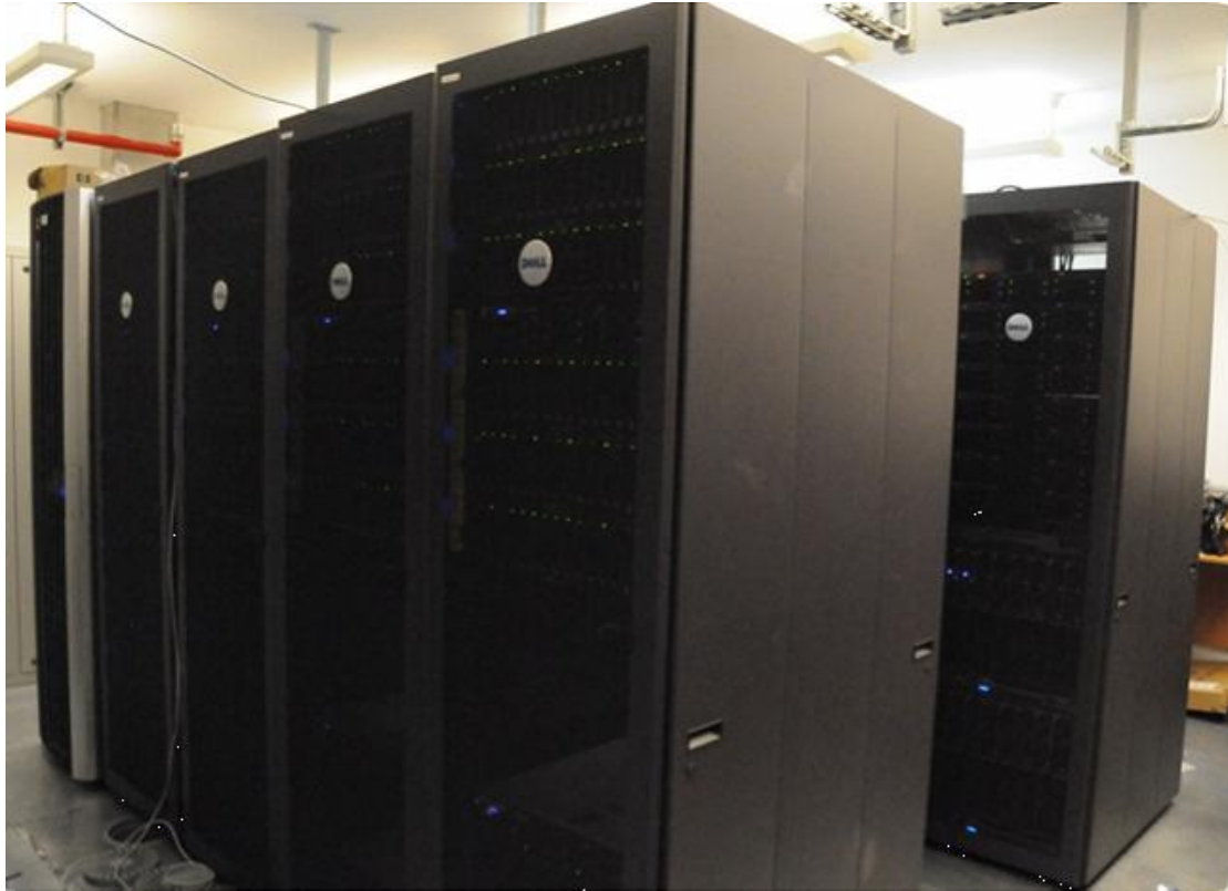
Figure 4: csTCDie Datastore Racks Far left: ExDS rack, then left-to-right four MD1000 racks
