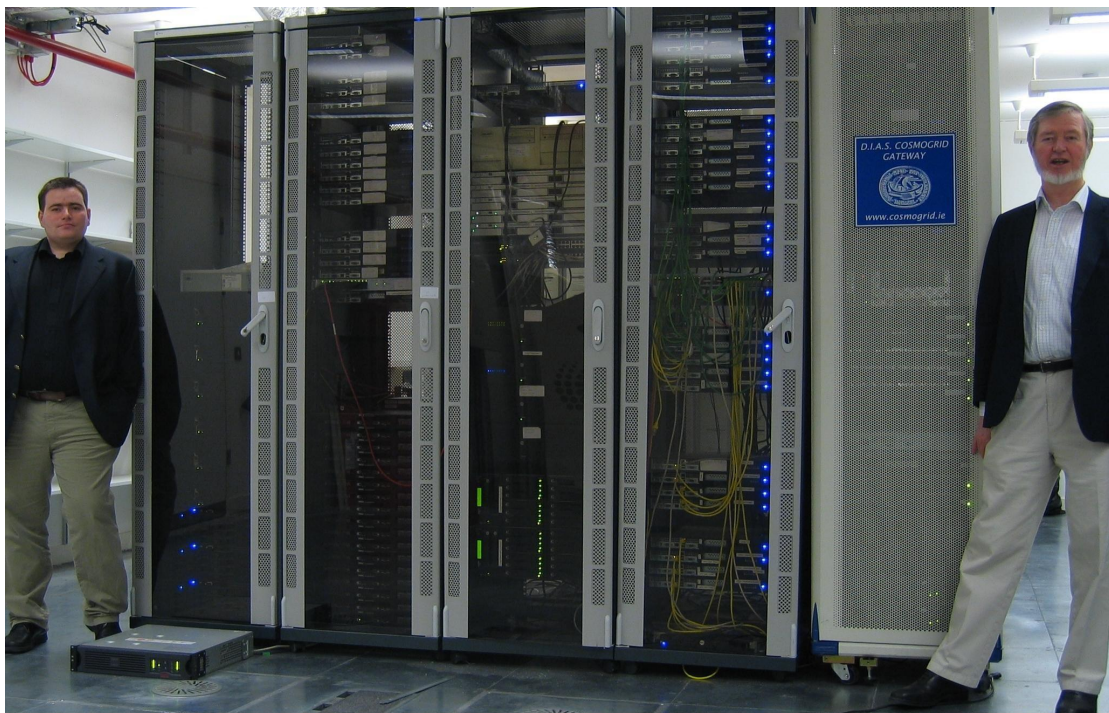
The Operations Centre machine room at TCD
