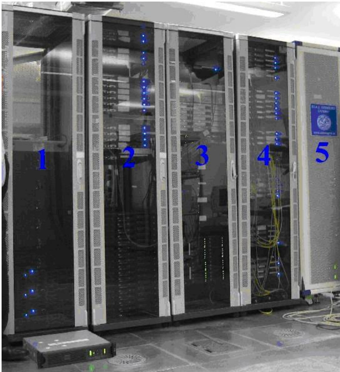
The Operations Centre machine room at TCD
